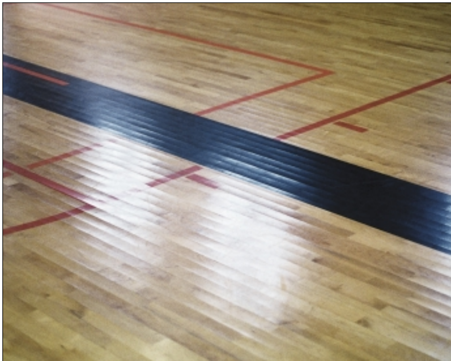
Excessive moisture in the interior environment or from beneath the floor can cause wood flooring to take on moisture. The result can be a "cupped" floor. For more on cupping, see page 19.
